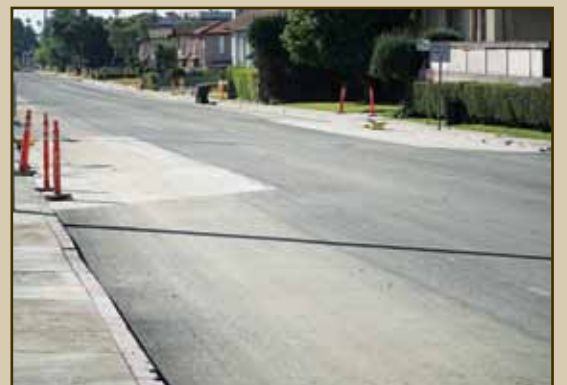
By this time, construction crews have completed placing the final layer of asphalt. The concrete pad on the left is designed for a bus stop. Because asphalt is a flexible material, this bus pad will allow buses to load without impacting the rest of the street.
