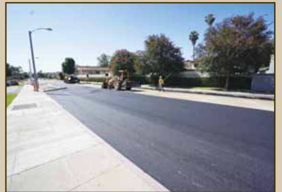
After preparing a new subgrade, construction crews are now laying down the initial layer of asphalt known as the base. Another layer of asphalt will be placed on top of the base before crews begin striping the road.
