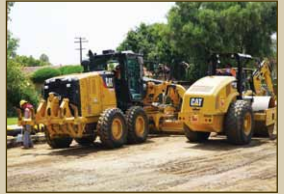
Here, construction crews are tearing out two layers of asphalt and one layer of base as Mission Road prepares for reconstruction.
